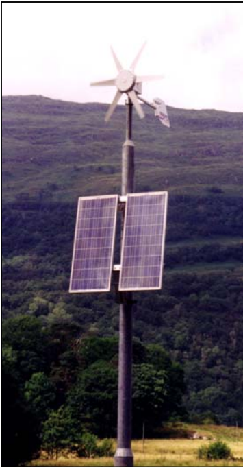
A low energy remote power site where a grid connection would otherwise cost thousands of pounds
